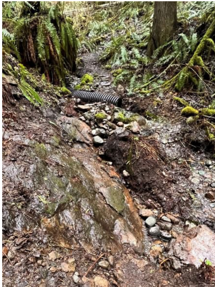
Water damage on the Phil's Creek Trail on Squak Mt.
